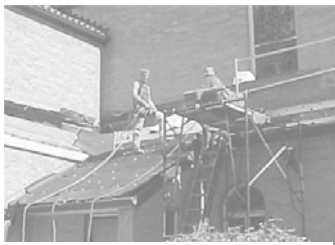
The clay roof tiles are removed to make repairs to the underlayment.
