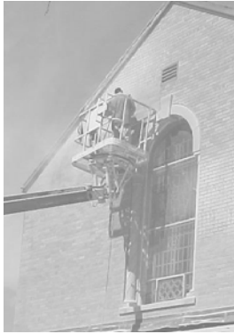
The mortar between the bricks is drilled out and will be replaced to seal the exterior walls.
